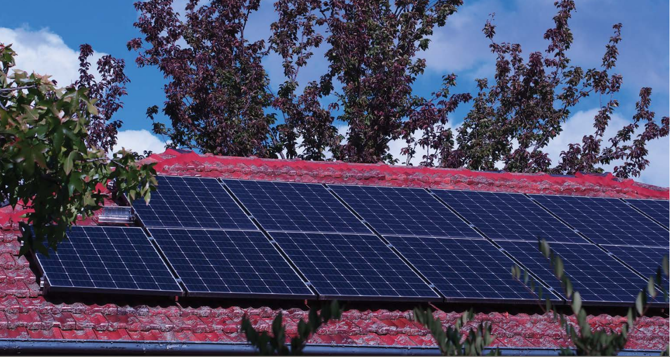
Residential rooftop solar panels. Photo: Jonathan Mandl, Clean Energy Regulator.
