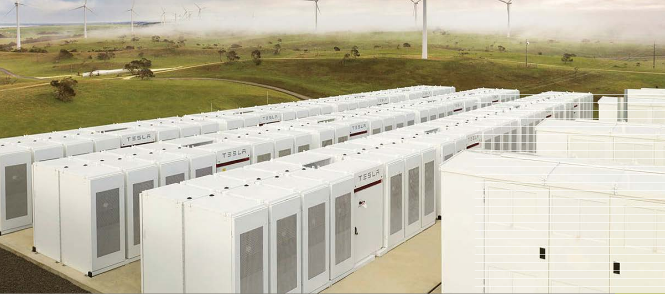
Tesla battery installation at the Lake Bonney Wind Farm in South Australia. Photo: Infigen Energy.
