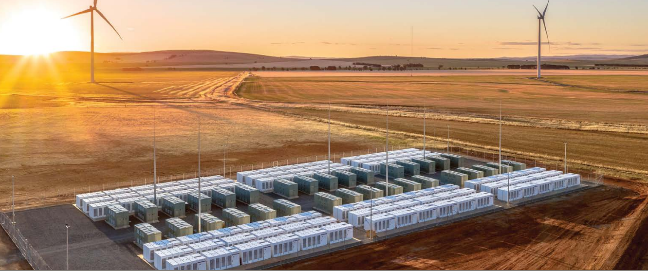
Hornsdale Power Reserve – a grid-connected energy storage system co-located with the Hornsdale Wind Farm. Photo: Clean Energy Finance Corporation.
