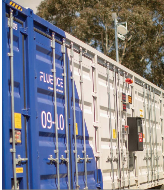
Ballarat Energy Storage System. Photo: Consortium comprising AusNet Services, Spotless, EnergyAustralia and Fluence.
