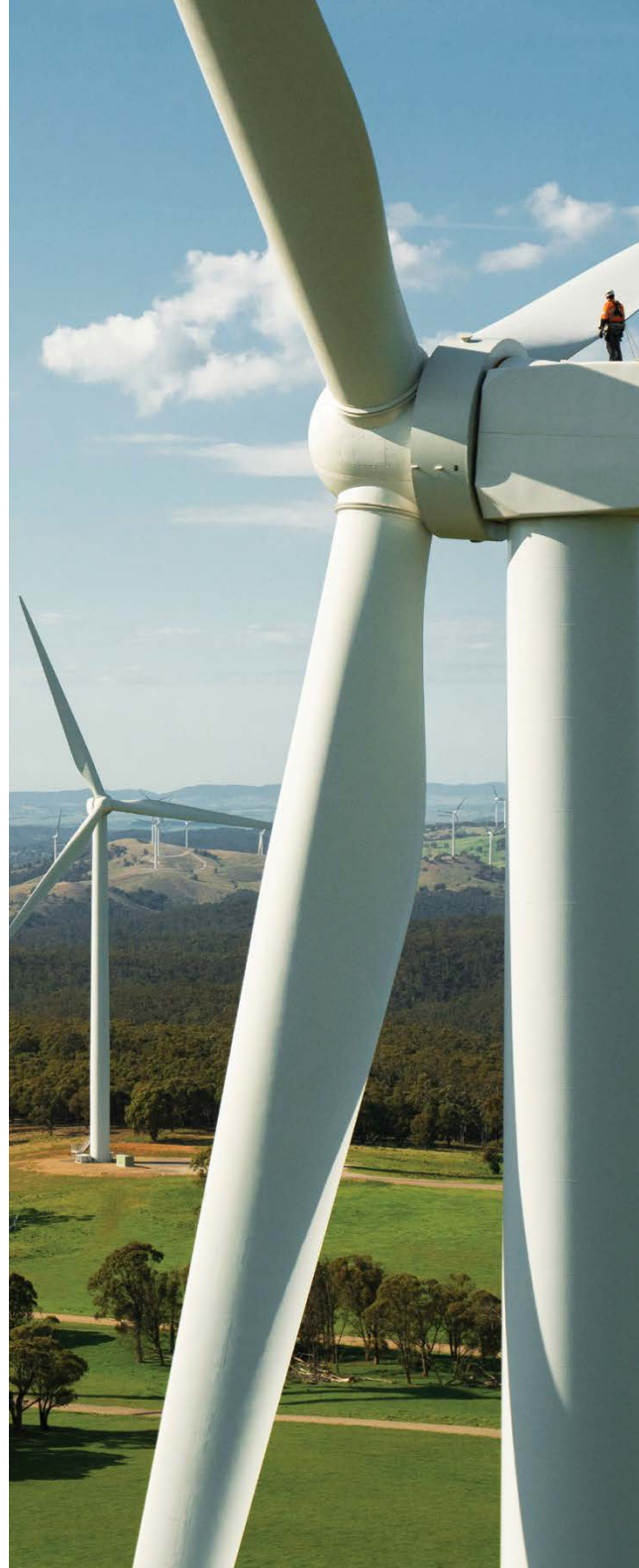
Maintenance check on wind turbines at Gullen Range Wind Farm, NSW. Photo: BJCE Australia.
